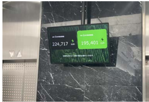
Digital signage installation (Daiwa Ginza)
