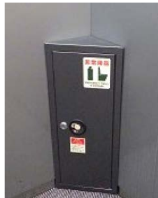
Elevator emergency goods box (Daiwa Azabu Terrace)
