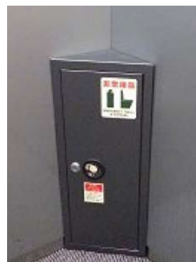
Elevator emergency goods box (Daiwa Azabu Terrace)
